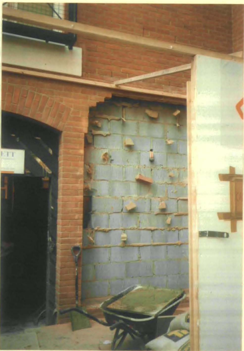
Photo 3 New Louvre in Courtyard of Willoughby St. Elevation 'B' in 06/B
