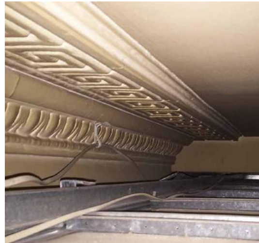
Fig. A25 Original cornice rear room ground floor (above modern suspended ceiling)
