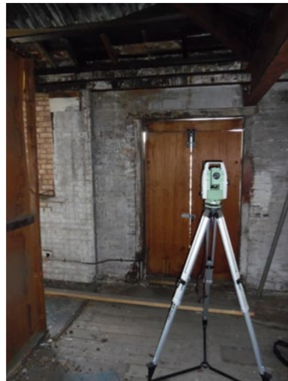
5. Structurally unsound floor
