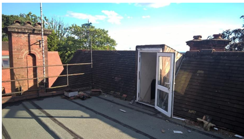
Figure 4.2 View from flat roof of one of the pitched sections of roof showing small number of broken tiles
