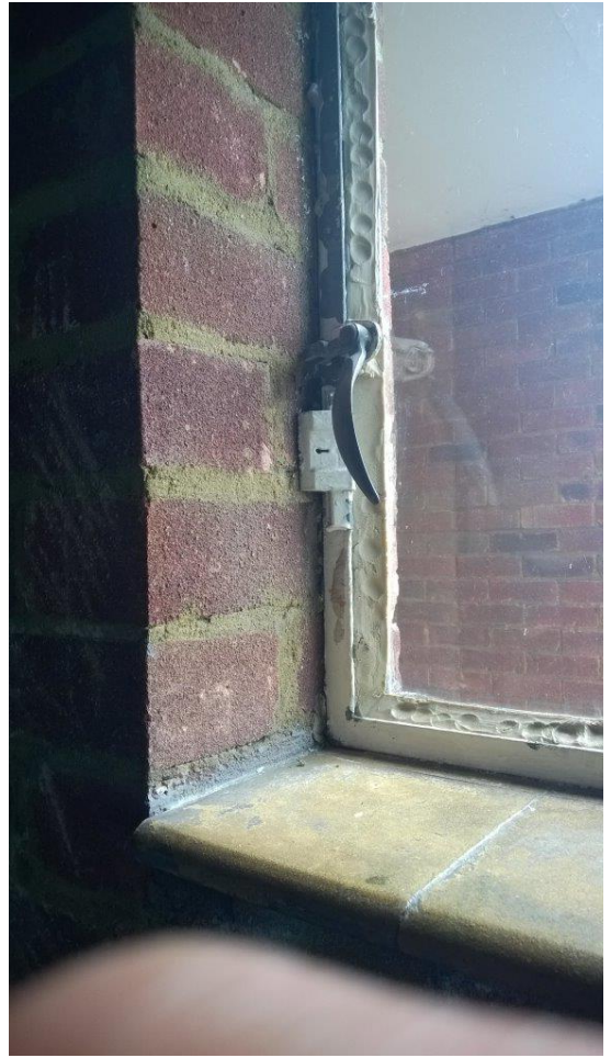
INTERNAL HANDLE AND DEFECTIVE PUTTY
