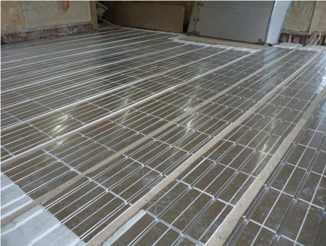
With average 400mm centred existing joists it was possible to install 3 pipes in per void resulting in optimum heat output.
