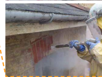
Proposed paint removal technique - Poultice type system to lift the paint from the brick fascia, followed by cleaning with a Doff system or similar approved - subject to testing
