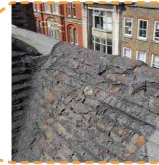
Original roof to No. 6 Denmark Street - in poor condition but revealing clay tiles - period correct
