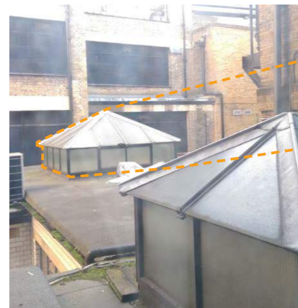
Existing roof lanterns and roof covering showing poor condition
