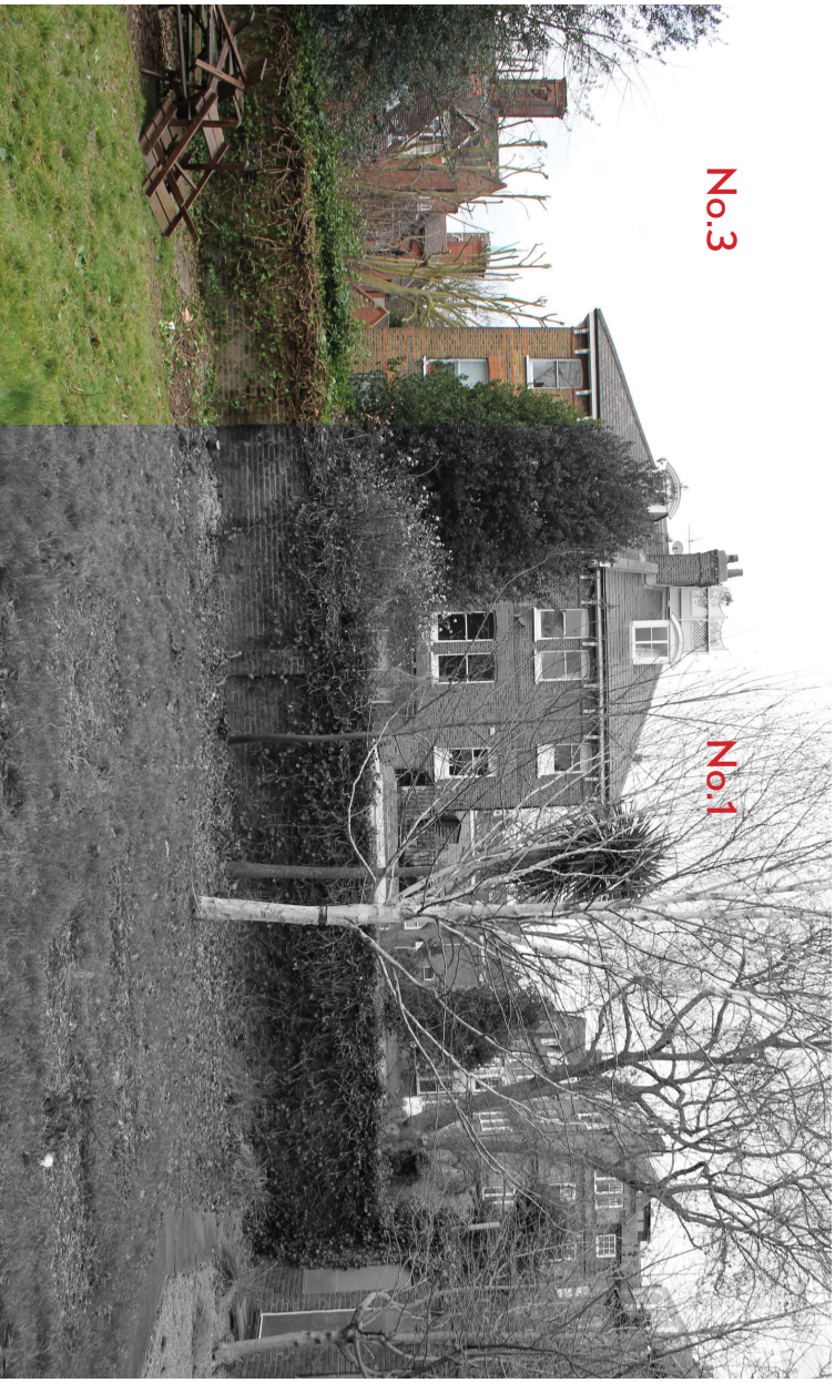
Images to the right show views of the existing northern boundary wall between the site and No.3 Ellerdale Road. Wall to be rebuilt.
