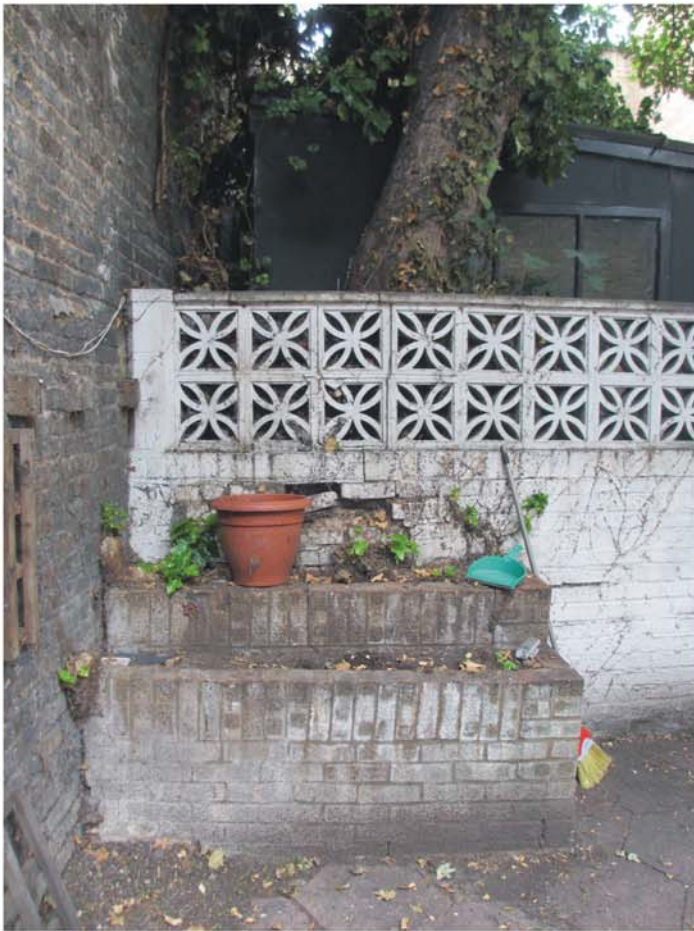
Photograph 7. View of the subject tree looking to the west showing the damage to the boundary wall.
