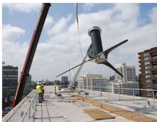
A building-mounted 6kW Proven wind turbine
