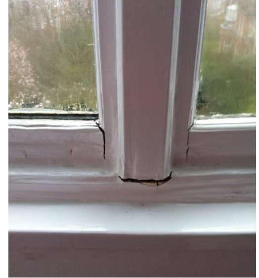
View 3 of the damaged window
