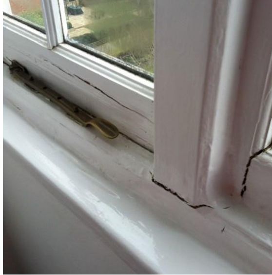
View 2 of damaged window
