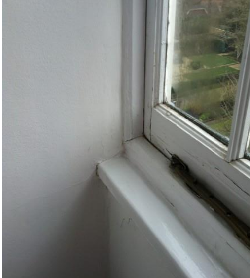
View 1 of damaged window
