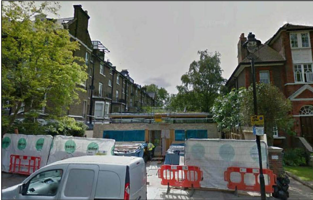
View to Rear of 15 Elsworthy Terrace with the approved scheme under construction
