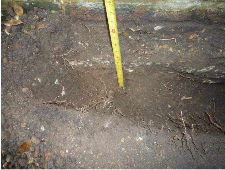
1) Trial trench showing a few small roots growing under the wall foundation.
