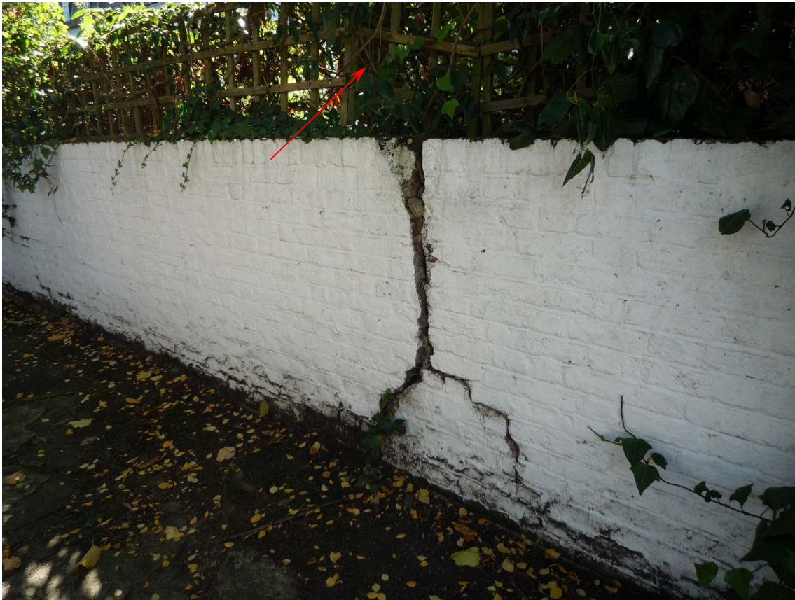
4) crack in the side wall seen from in front of no.23. Arrow shows the birch trunk.
