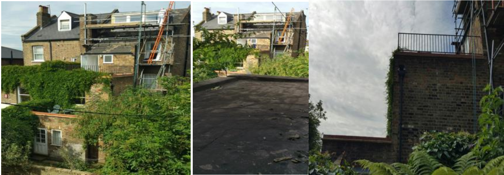
68 Marquis Road double terrace extension from both side and rear view from existing terrace at 81 York Way
