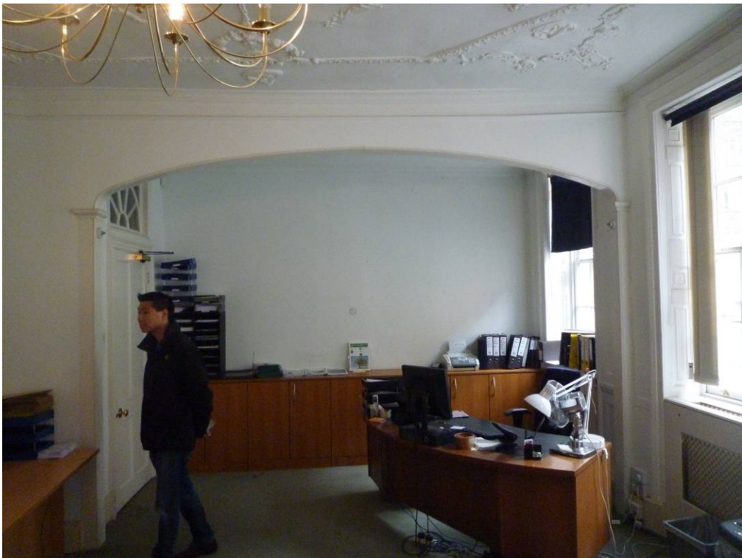
Fig. 38 Ceiling in first floor front room from the north, showing the modern archway
