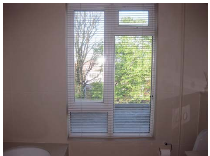
Existing constrained view from first floor bathroom window
