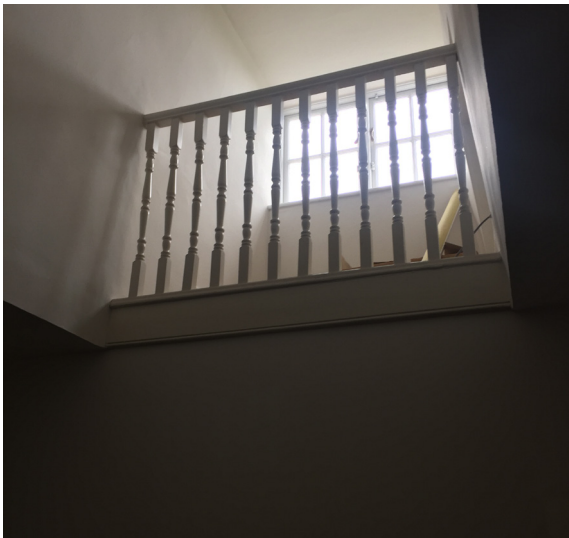
Fig. 6_ No access to balcony or window
