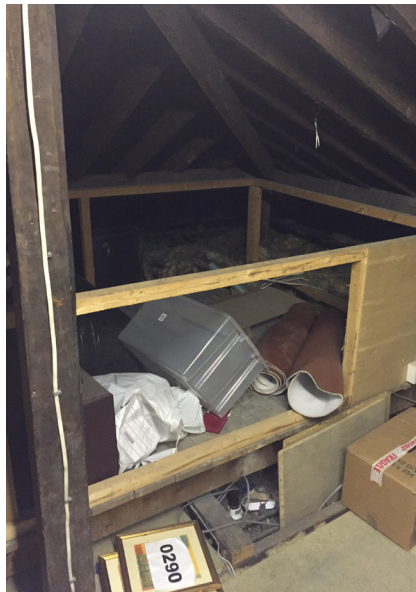
Fig. 13_ Redundant water tanks in loft
