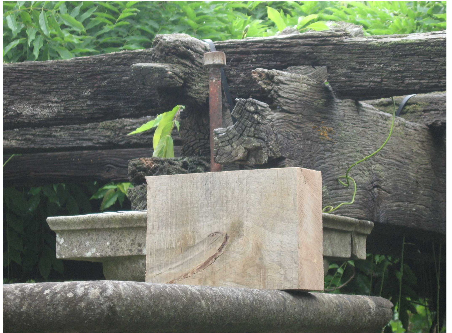
Photo of seasoned English Oak sample against 1911 oak beams and joists in the Pergola Colonnade extension. Note existing wet timber dark colour due to rain water darkening the oak. The sample instead is completely dry oak.
