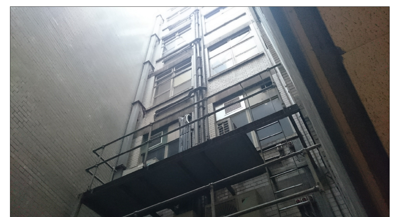
SITE PHOTO OF EXISTING SOUTH ELEVATION TO LIGHT WELL (FROM GROUND FLR)
