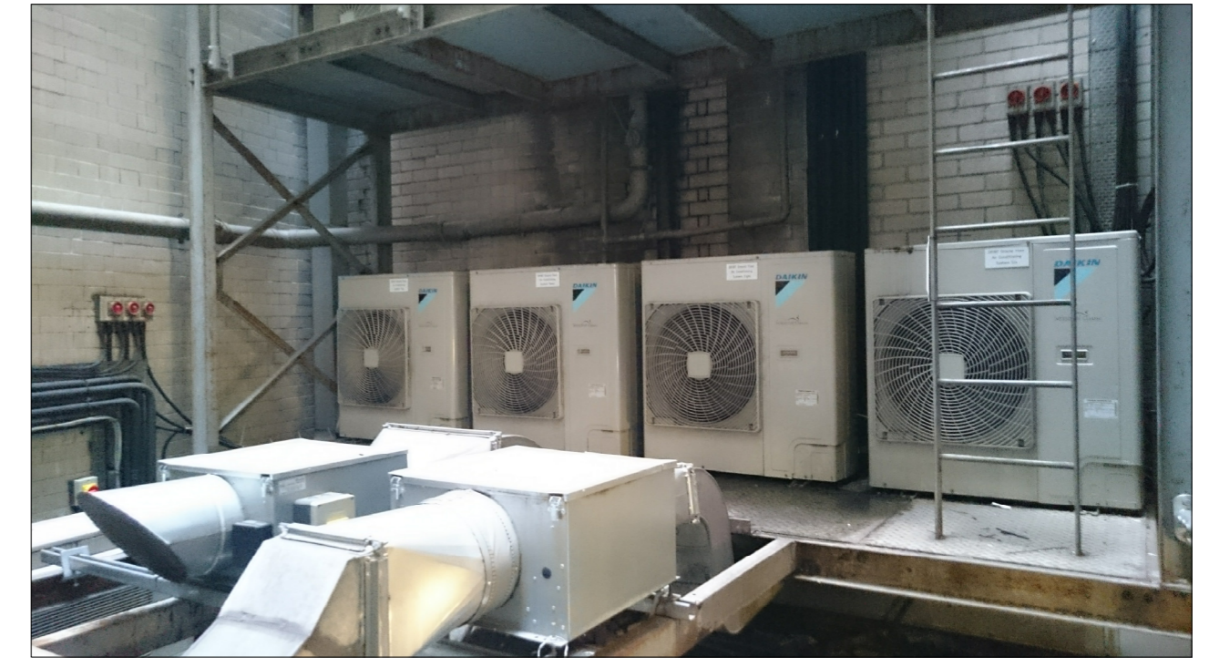
EXISTING PLANT SERVING RETAIL UNITS - GROUND FLOOR
