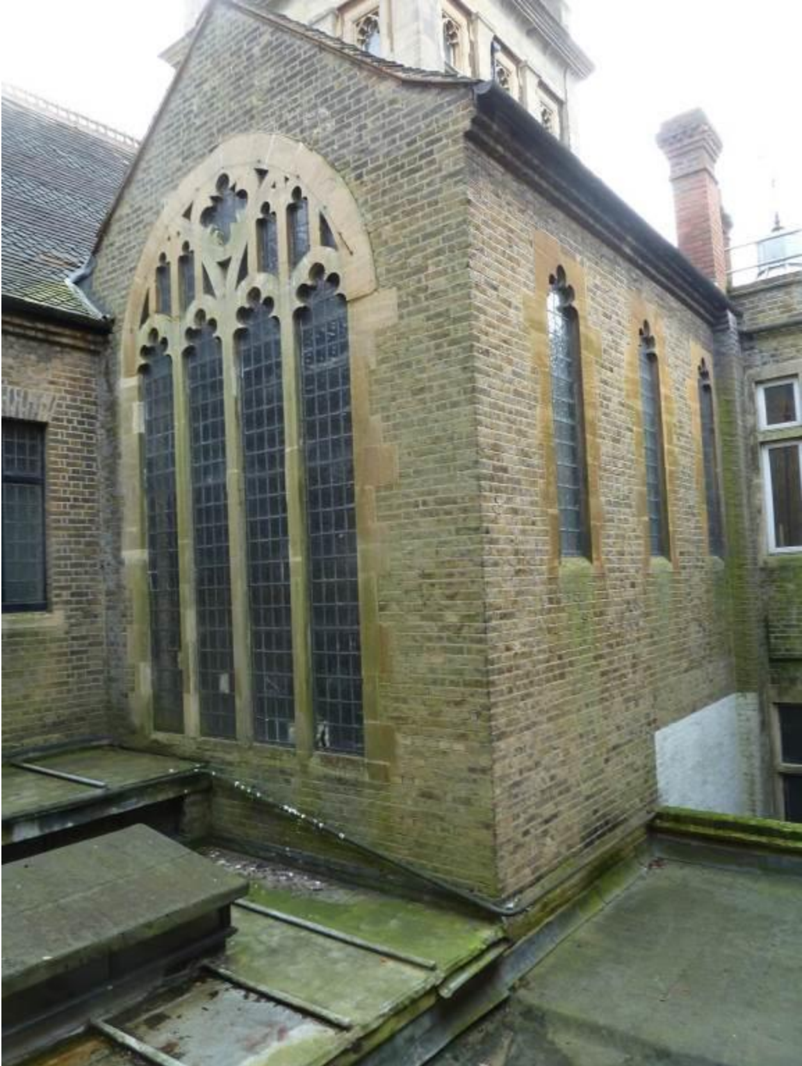
MMP48 Exterior of Great stair showing use of London Stock Bricks. The ground floor buildings are to be cleared to create the atrium and the external well in which the window wall will be exposed (March 2016)
