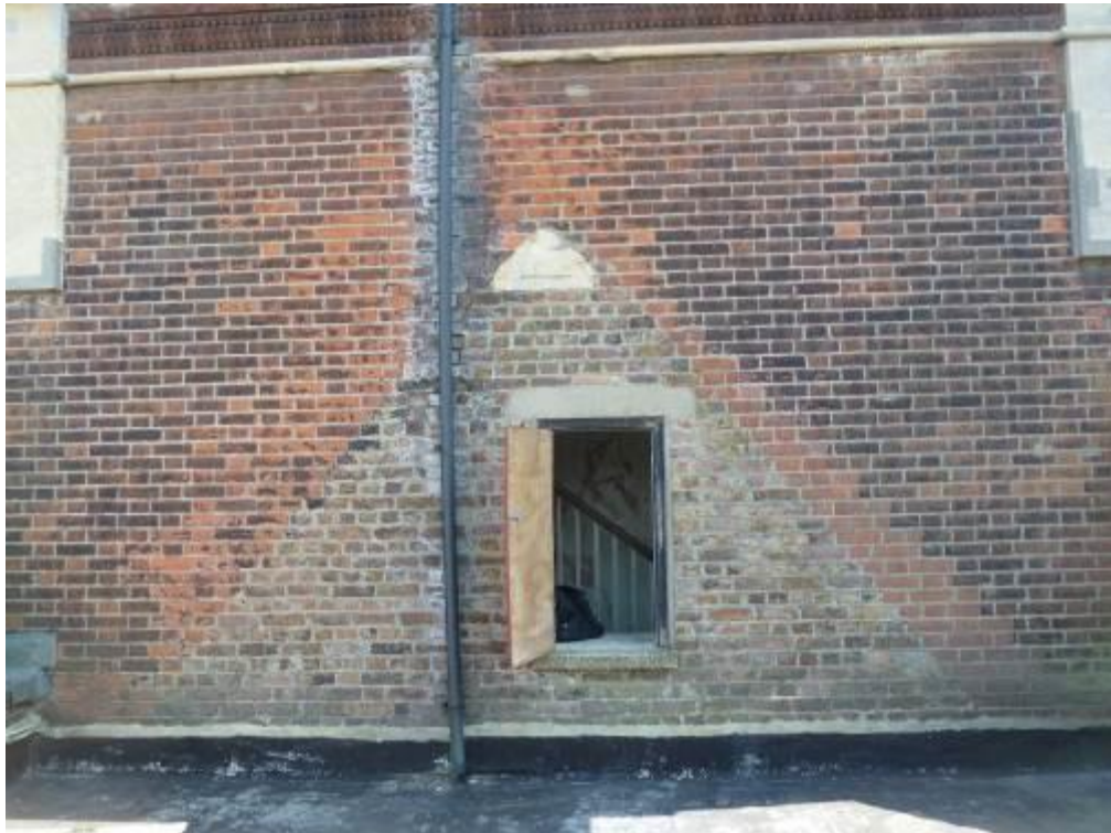
MMP42 Profile of demolished roof (post 1948) and change to London stock brickwork in original attic space on rear wall of tower (August 2014)
