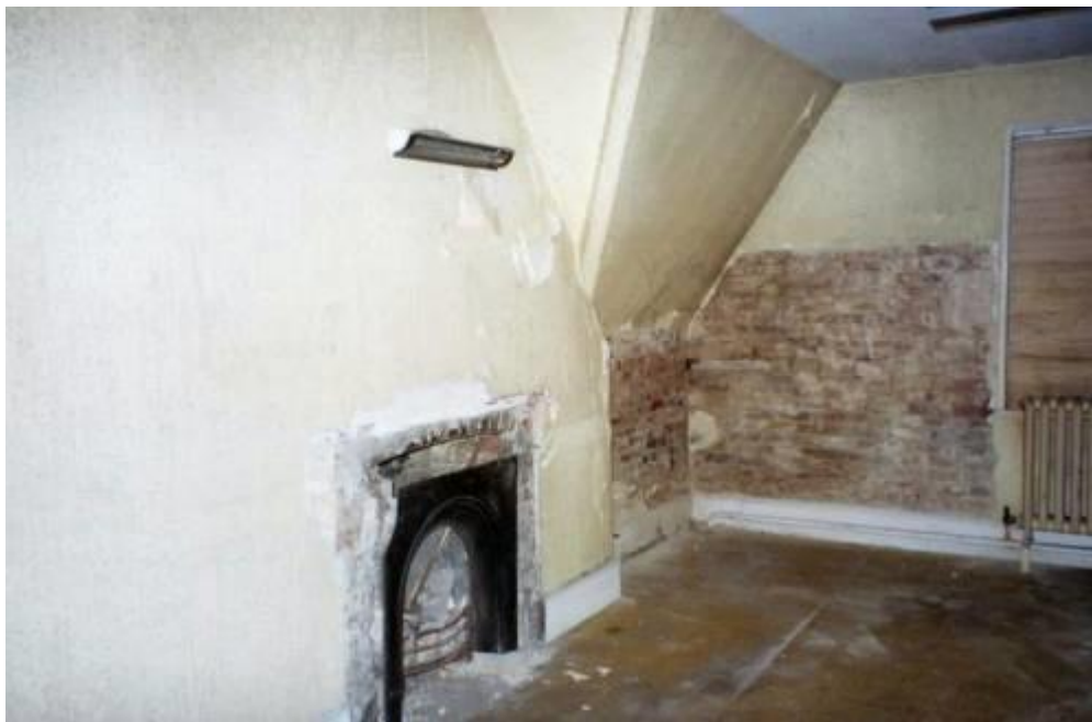
MMP28 Derelict and vandalised attic servants' bedroom
