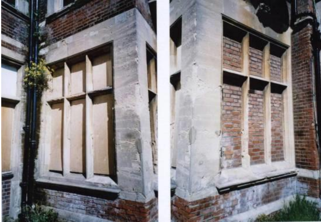
MMP11,12 Decay of Morning Room windows, particularly mullions on South Elevation
