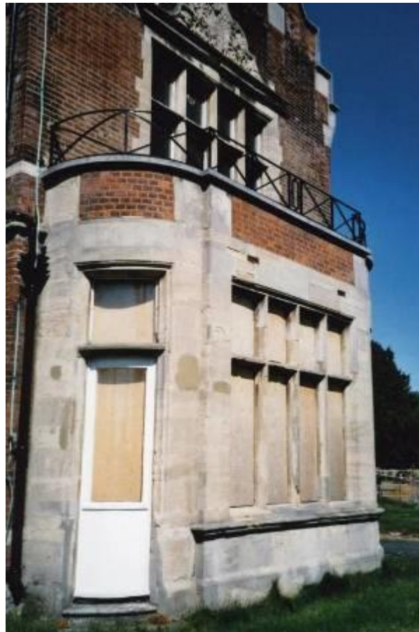
MMP17 Cement patched and decayed stonework of Billiard Room bay window
