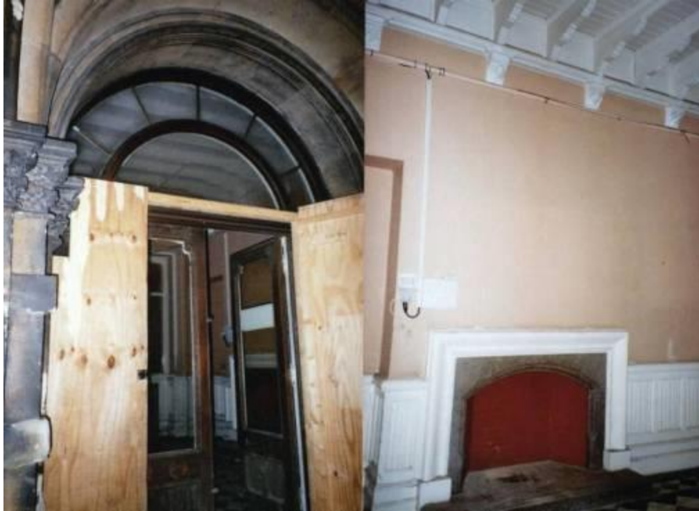
MMP26, 27 Entrance from Porte Cochere and Ante Hall with fireplace and dado, cut profiled joists and carved stone corbel blocks (painted over).
