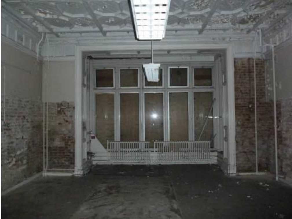
MMP 46 Dining Room looking into bay window; note painted boarded ceiling (March 2016)
