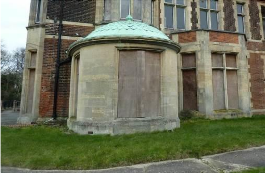
MMP44 Pavilion extension c. early 1900s (August 2014) to be demolished as approved in 2005
