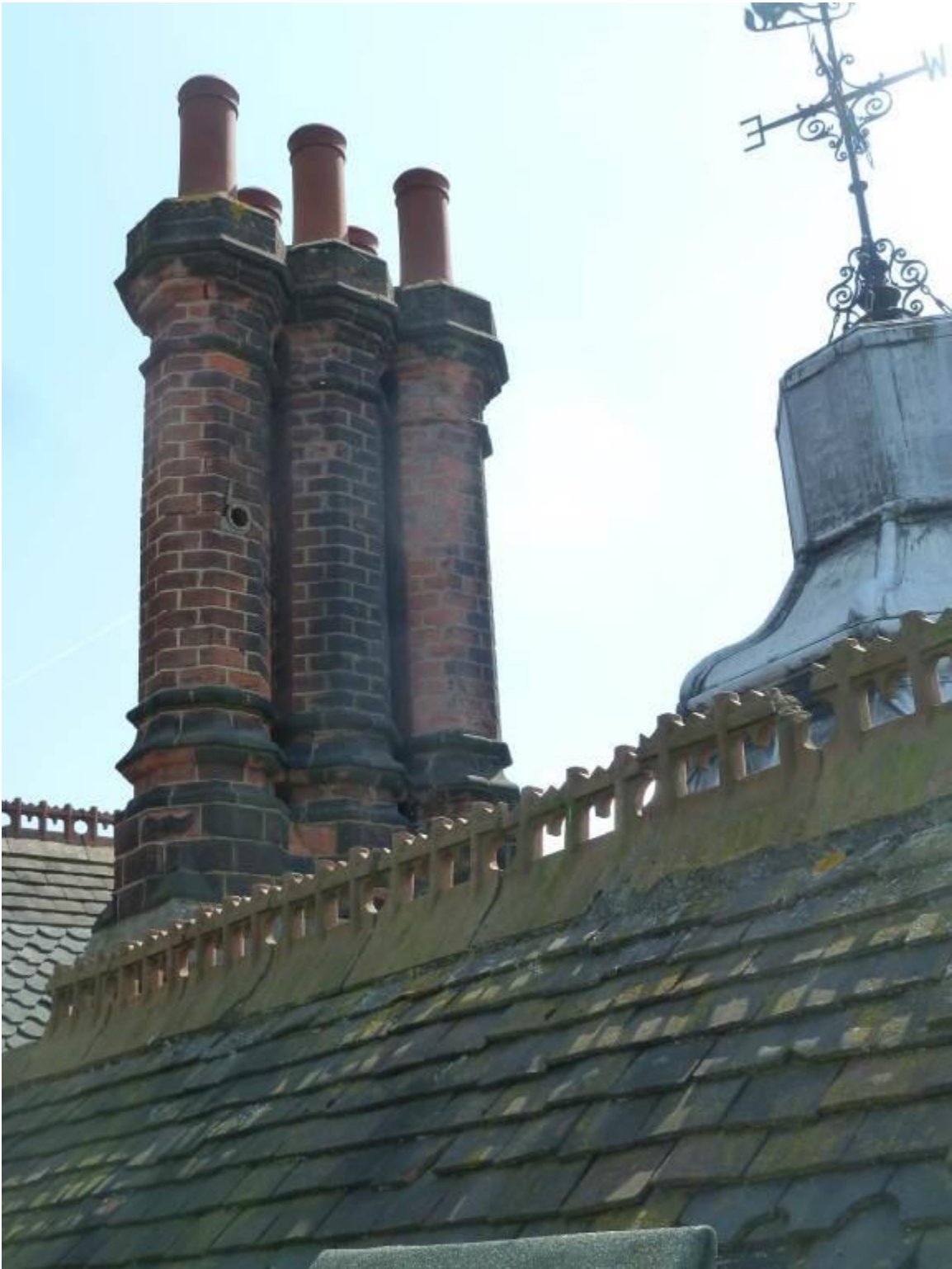
MMP43 Cluster of original chimneys behind cupola (August 2014). A glimpse of the 'Beaver' weather vane can be seen projecting from the cupola roof. The fretted ridge tiles may have been recently replaced, probably within the last 20 years.
