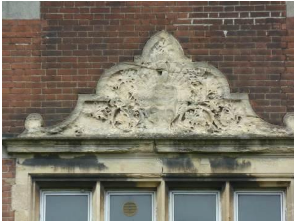
MMP 53 Eroded 'Peacock and Foliage' panel above right hand first floor window, south elevation, compare with MMP 9, 10 above (March 2016)
