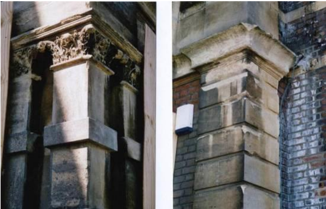
MMP13, 14 Eroded ornamental stonework on Porte Cochere
