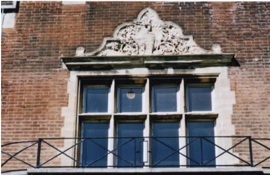
MMP9,10 Economy balustrade, simplified gable and eroded stonework of the South Elevation. The 'peacock and foliage' panel above the window has further deteriorated since 2007.
