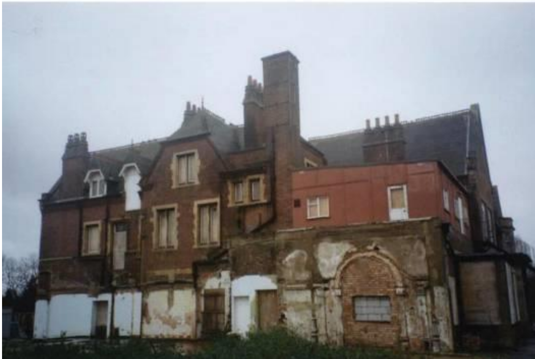
MMP 7, 8 'Hospital alterations' and the scars of demolition on the North Elevation, photographed in February 2007. The arched profile of the conservatory is clearly visible on the lower photograph.
