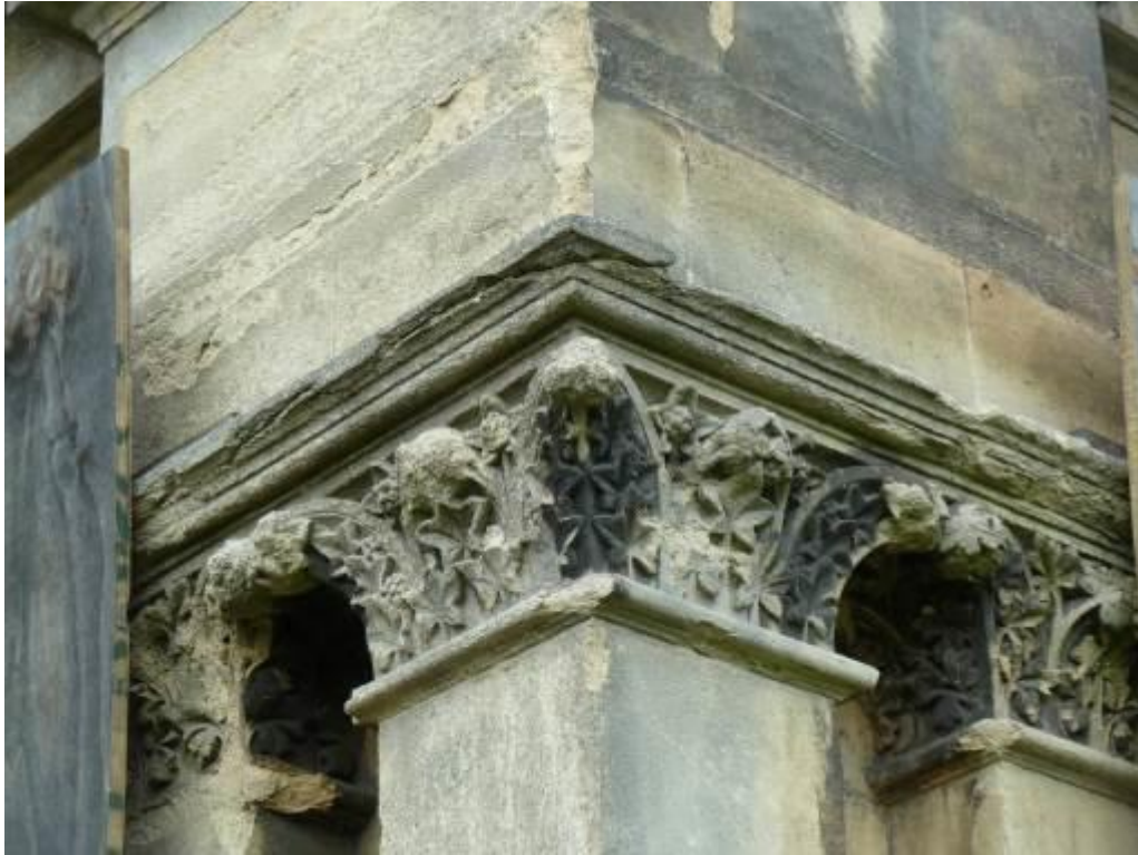
MMP51 Flaking stonework and carving on porte cochere (March 2016)
