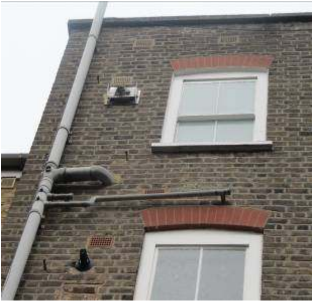
Frame No: 03 Location: Flat 3, 37 Lambs Conduit Street Description: Rear Elevation Date: June 2016
