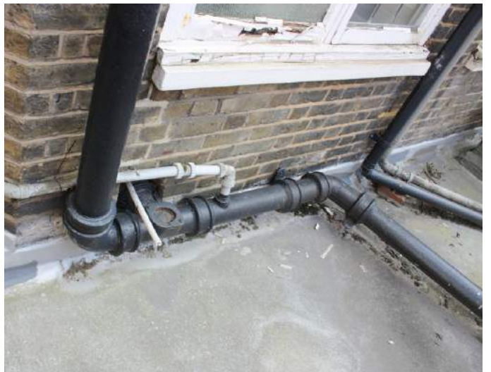
Lack of barrier at roof edge, windows to rear with rotten timberworkx.
