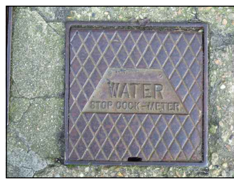
FIG 5 - STOPCOCK AND WATER METER COVER
