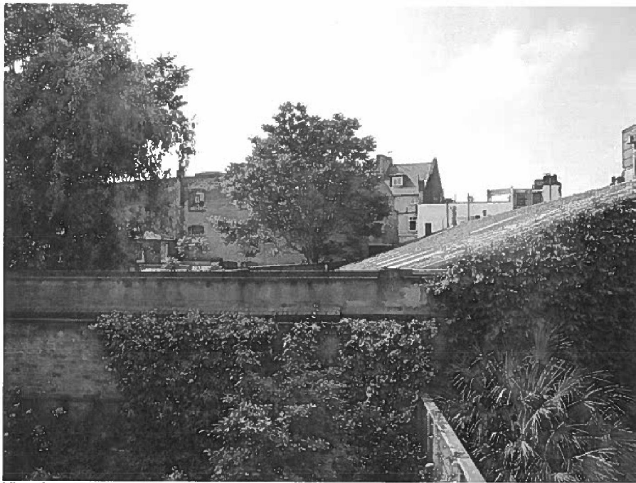
View from the rear of No.4 Collard Place showing flat roof and part of pitched roof
