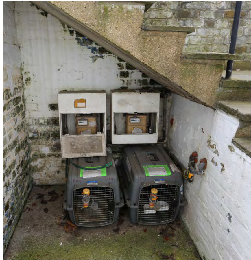
The light well to the front of the house is cluttered with incoming services. These are unsightly and despite being located under the stair they detract from the appearance of this external entrance.
