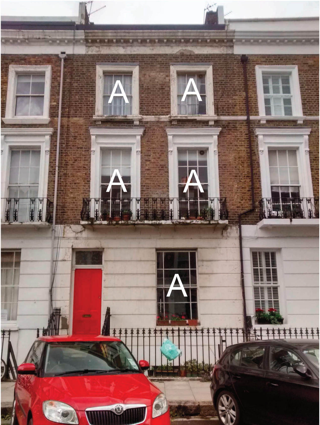
Street elevation windows to be replaced with new double-glazed timber windows (see drawing 254/11)
