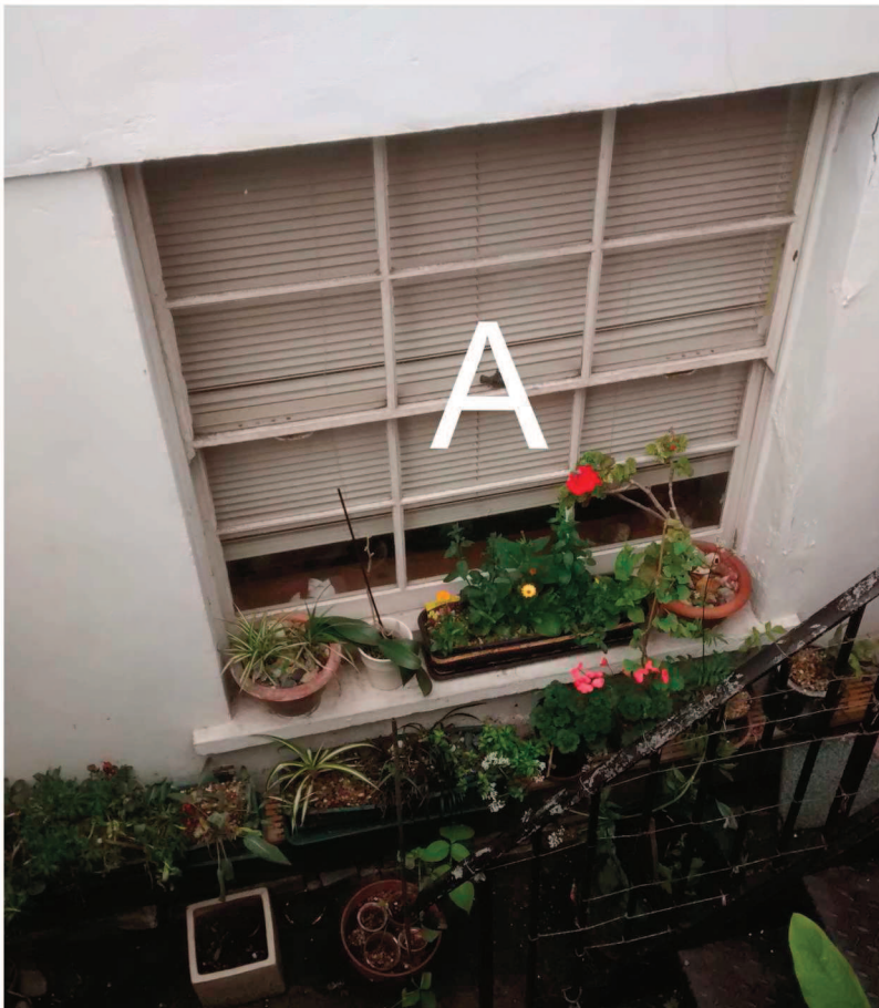
Basement window to be replaced with new double-glazed timber windows (see drawing 254/11)
