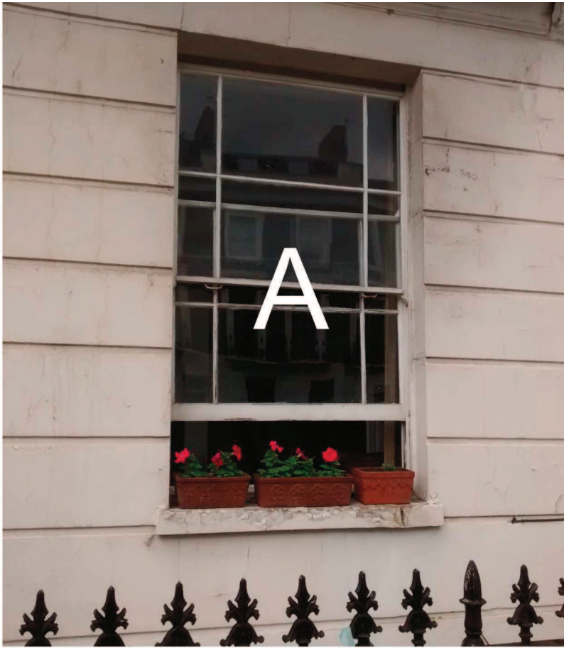
Ground floor window to be replaced with new double-glazed timber windows (see drawing 254/11)
