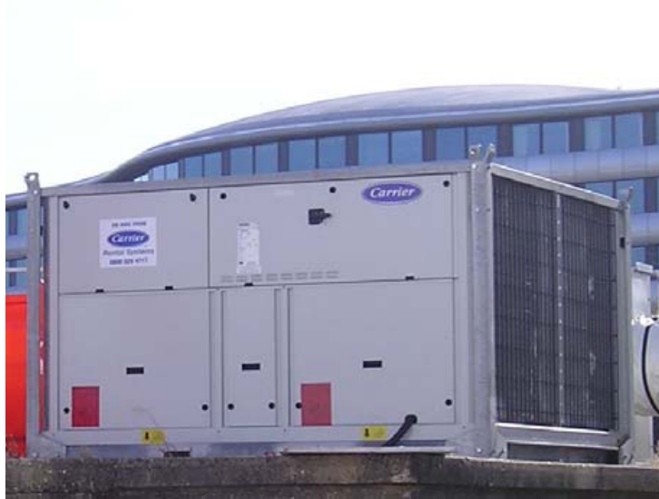
Chiller/ Heater Unit
