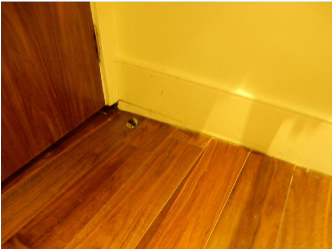
Photograph 9 – Previous repairs to dropped floor to cupboard under stairs. Infill installed to skirting.
