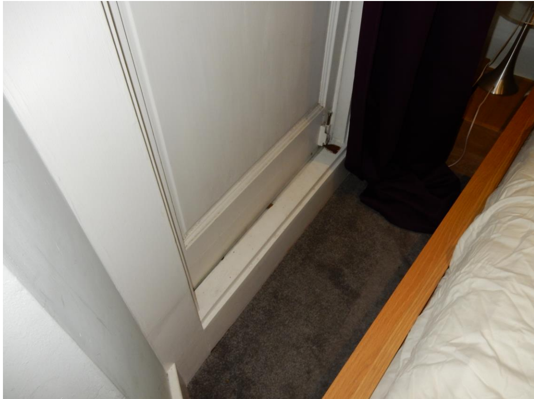
Photograph 7 – Front bedroom – External door not shutting properly. Adjustment required.
