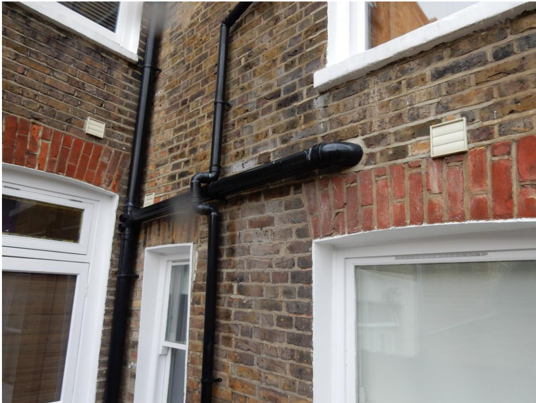
Photograph 10 – Rear and side elevation with brick spalling noted and evidence of previous repairs.
