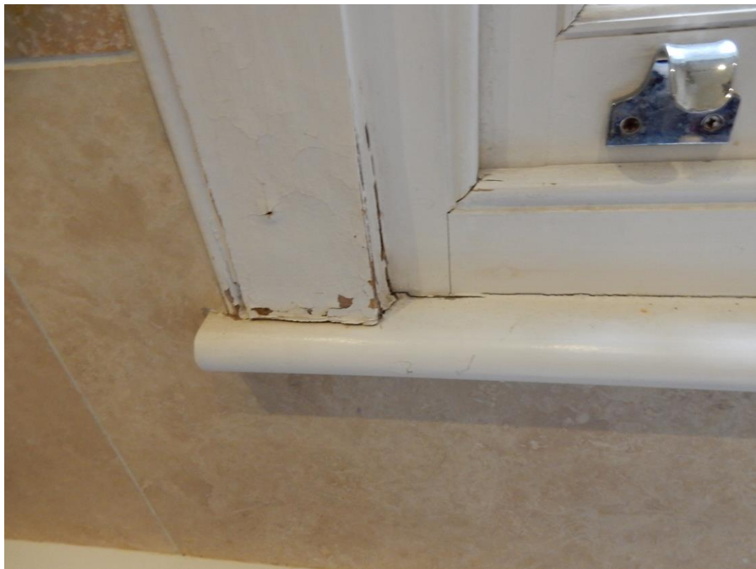
Photograph 6 – Main bathroom – Window above bath – Paint peeling and blistering.
