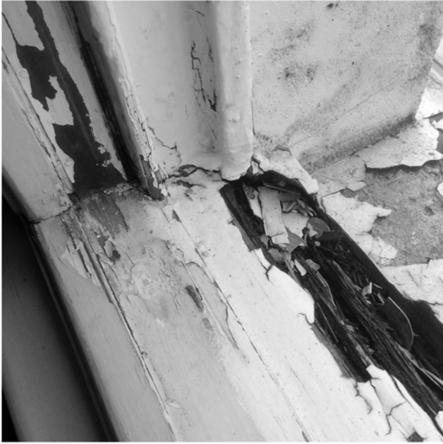
3rd Floor bedroom 1 window damage / rotten timber
