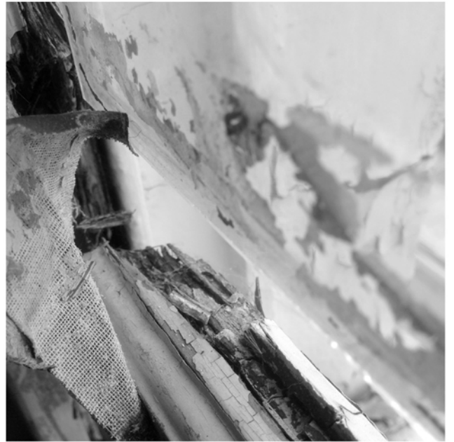
3rd Floor bedroom 2 window damage / rotten timber
