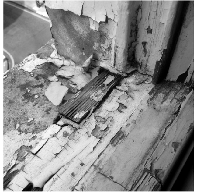
2nd Floor lounge window damage / rotten timber
