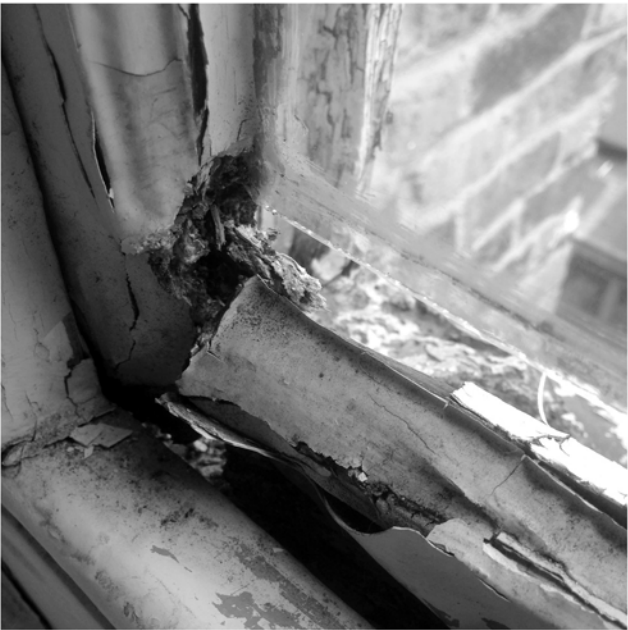
Stairs / Landing Window damage / rotten timber
