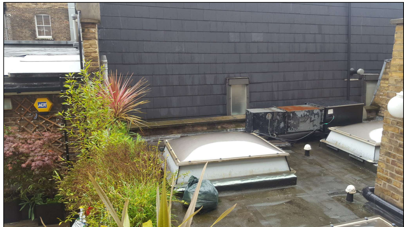
IMAGE 04- EXTRACTION UNIT AS EXISTING
