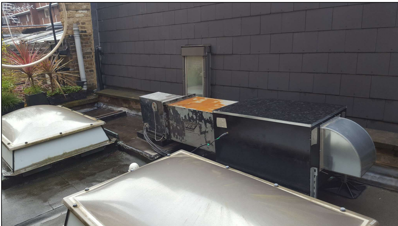
IMAGE 03- EXTRACTION UNIT AS EXISTING
