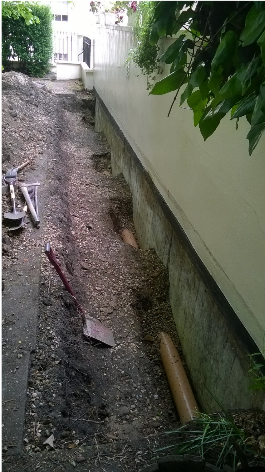
Photograph 1 – Hand excavated trench revealing no significant roots. Drainage pipe is lying on top of concrete foundation.
