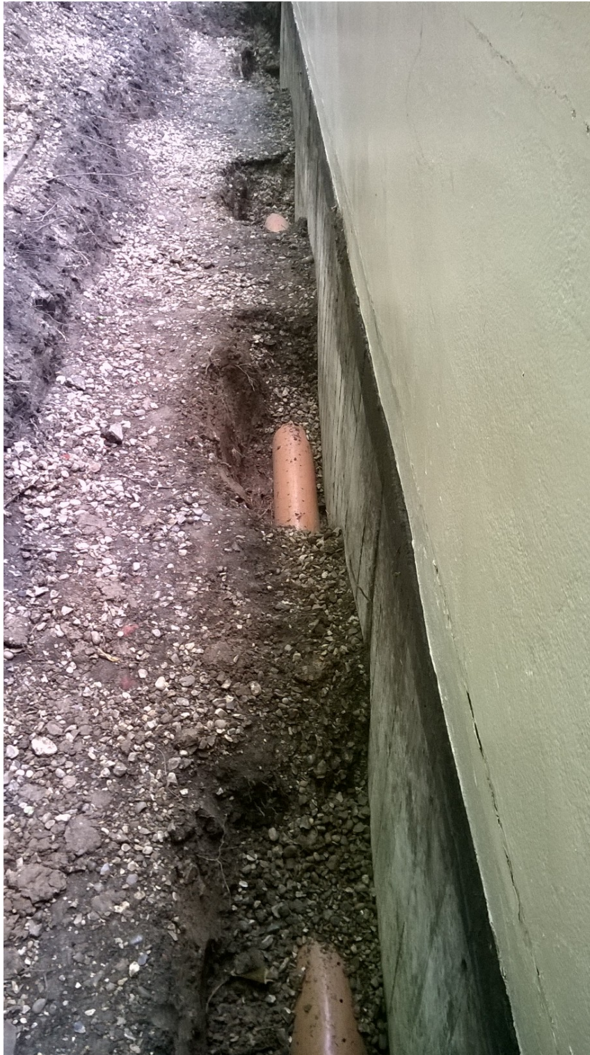
Photograph 3 – Some fine roots seen in upper soil horizons and in gravel/soil mix around drainage pipe.
