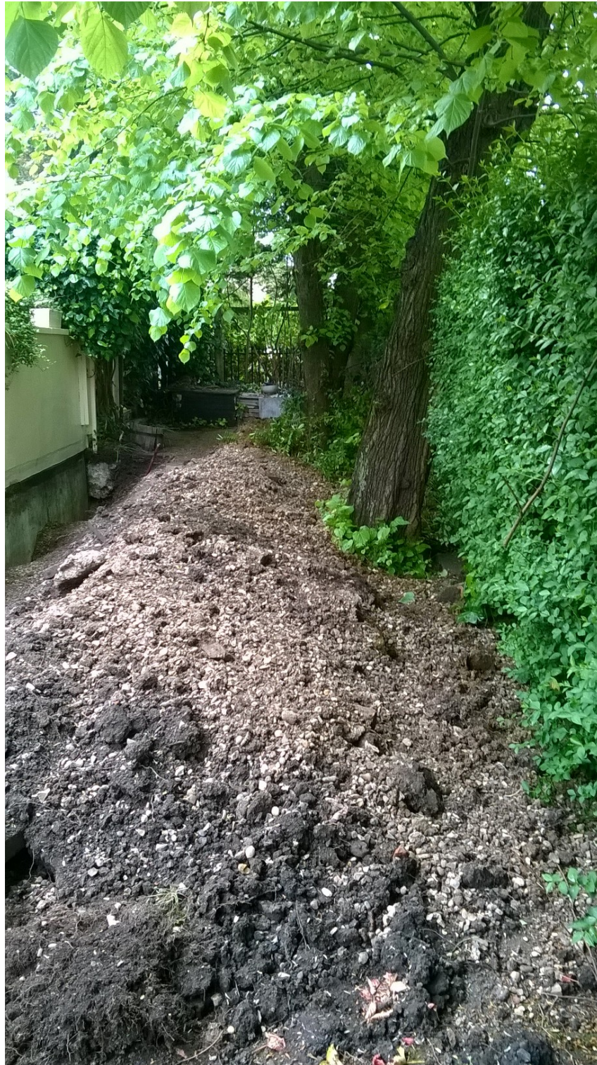
Photograph 2 – Temporary placement of soil excavated from trench. No severed significant roots in soil.
