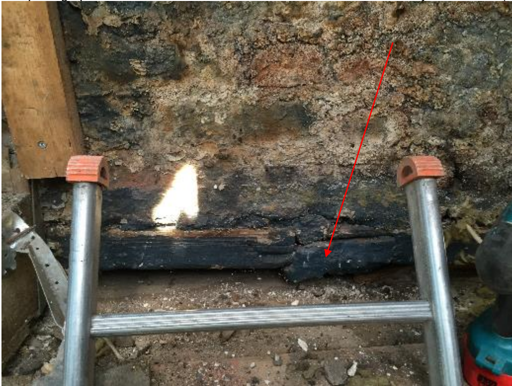
Photograph 4: Poor condition of the lintel observed over the doorway located on the east elevation. The photograph shows that the lintel has failed in service as illustrated by the fracture (arrowed).
