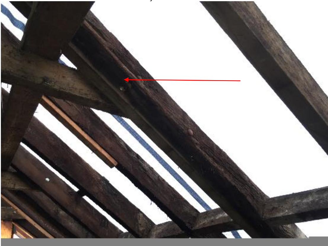
Photograph 12: An example of erosion caused by surface decay and loss in cross section observed on a common rafter as marked by the arrow.
