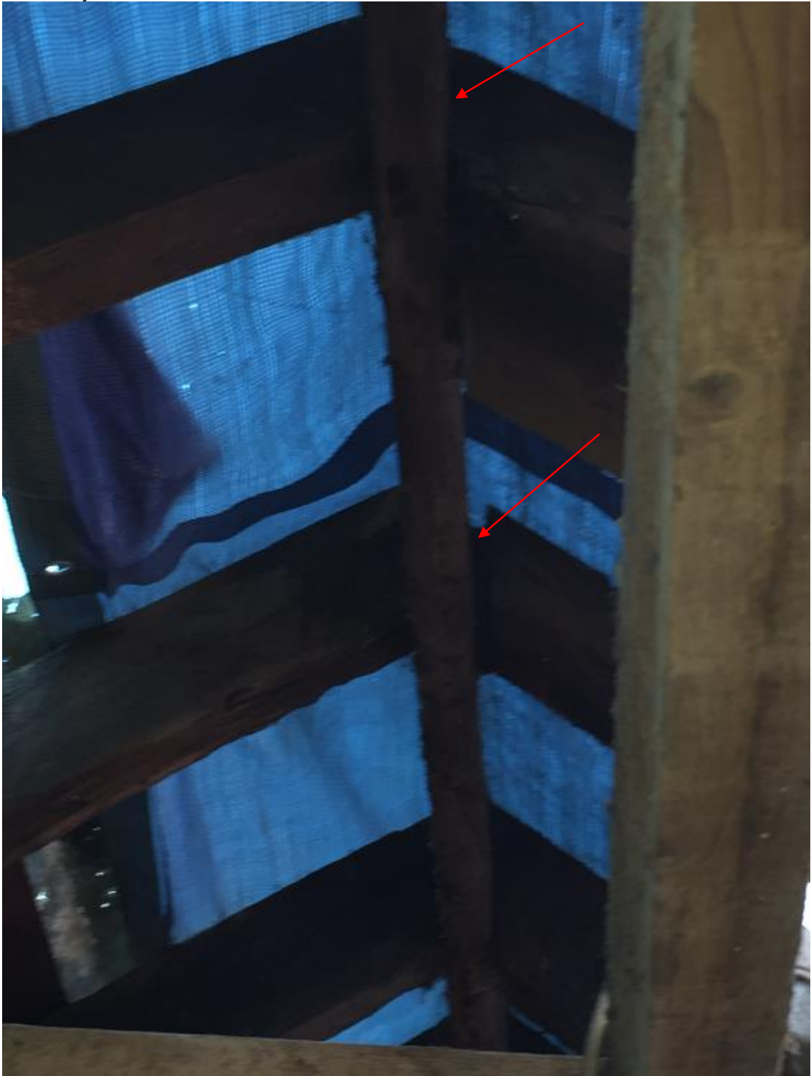
Photograph 10: Evidence of movement and dislocation of common rafters from the ridge as marked by the arrows.
