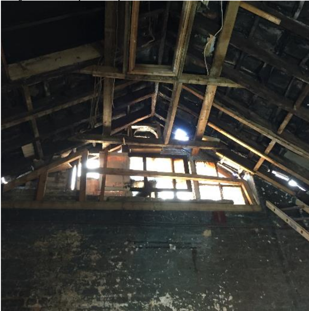
Photograph 9: Construction of the roof along the east elevation of the smithy. Also note the rooflight has been subject to many interventions and is in poor condition.
