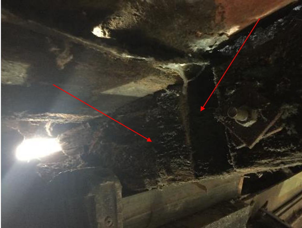
Photograph 7: Example of excessive notching (arrowed) observed on a number of the common rafters which affected indicative visual strength grade. Also note the chemical attack in the surface of the common rafter resulting in a woolly appearance caused by defibrillation of the outer layer of timber (arrowed).
