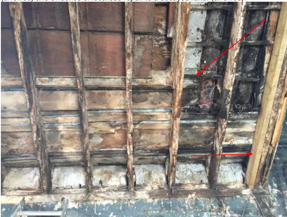
Photograph 8: Close up view of the front elevation of the smithy (Denmark Street) illustrating the common rafters bearing onto a timber wall plate. Also note the severe decay in the roofing battens (arrowed) and evidence of localised repair to a decayed rafter (arrowed).
