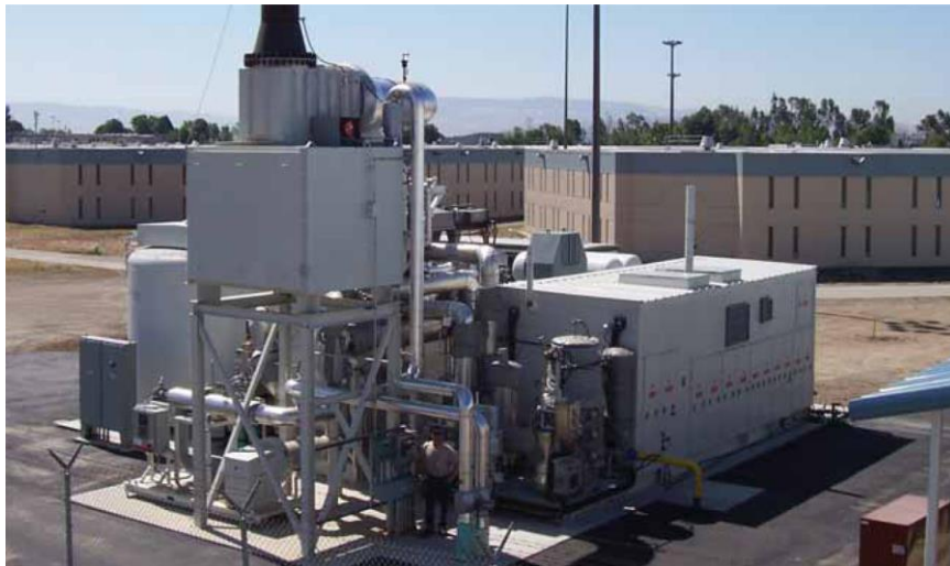
Figure 8: Example Fuel Cell Installation
