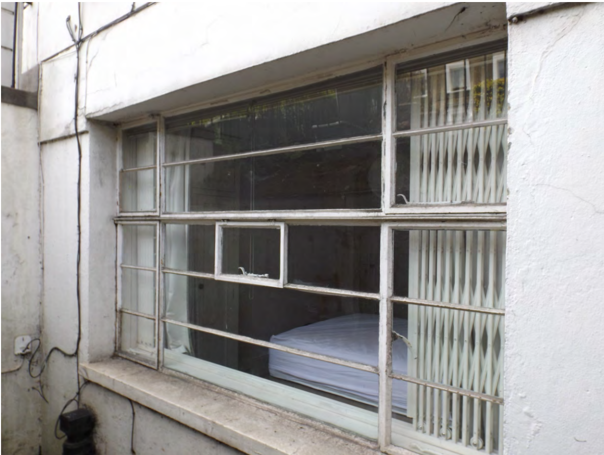
Appendix 1.2: Crittal casement window to be replaced
