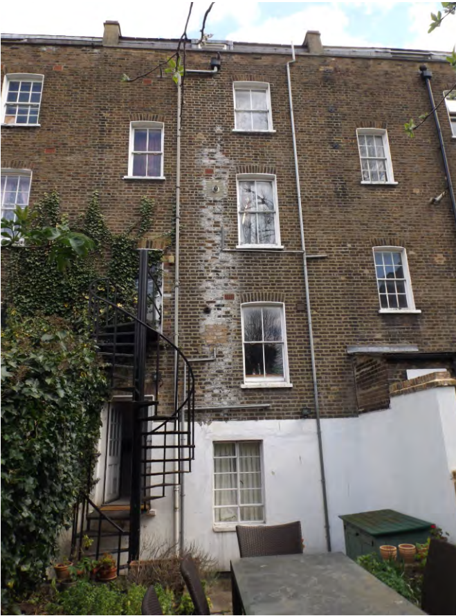
Appendix 1.3: Window at basement level and door to be replaced.
