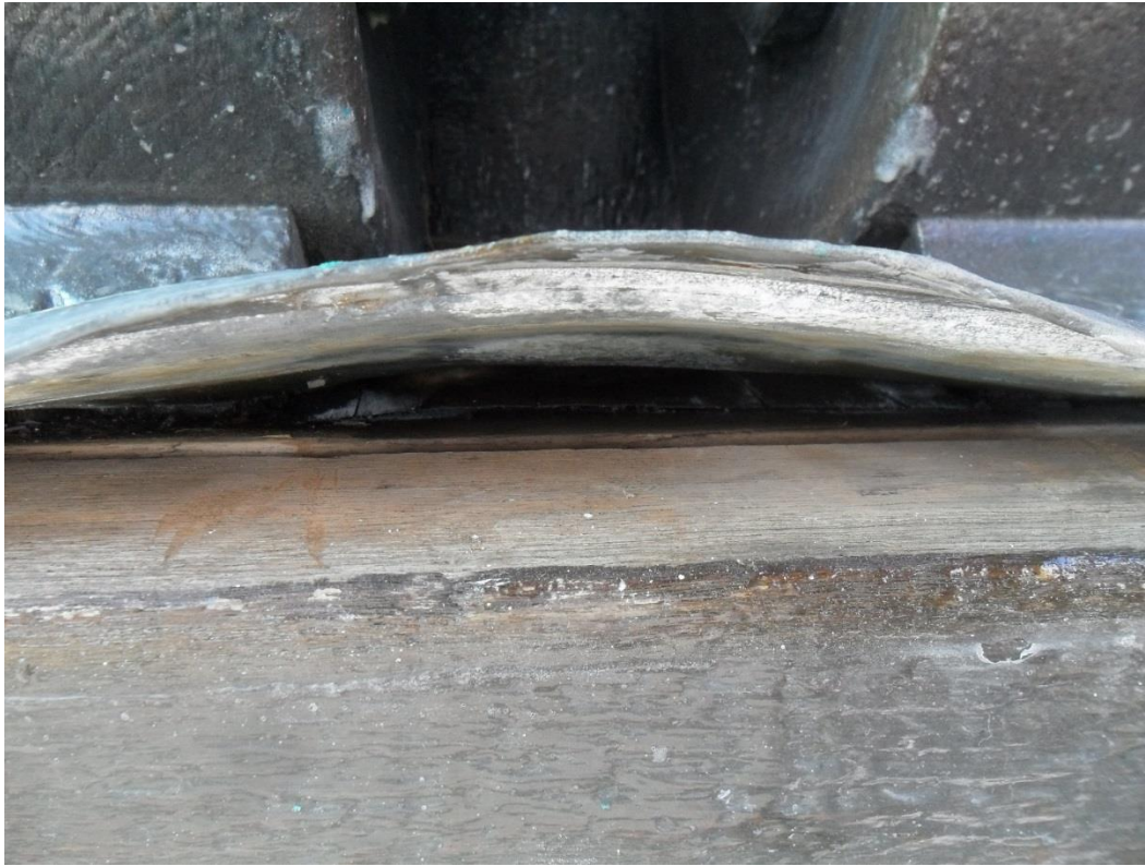
3) Close up of timber plinth immediately beneath scrolls with lead capping lifted. This shows the vulnerability of the plinth to leakage due to the built up construction.
