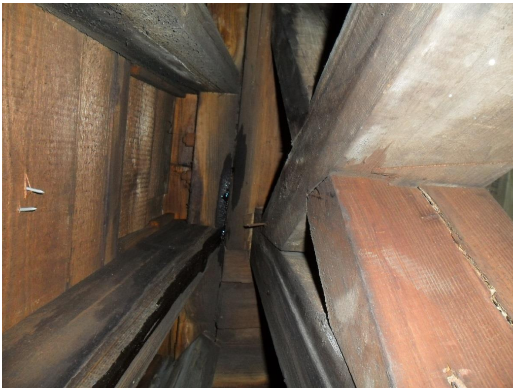
4) Typical leak beneath scroll plinth (looking upwards).
