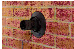
BOILER FLUE TERMINAL
