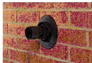
BOILER FLUE TERMINAL
