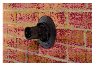
BOILER FLUE TERMINAL
