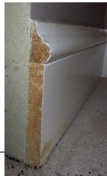
Existing skirting from room 3.03
