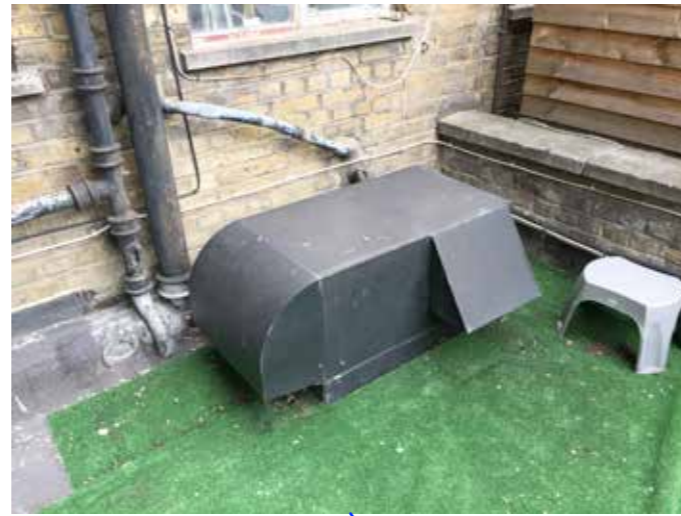
ROOF VENTILATION UNIT
