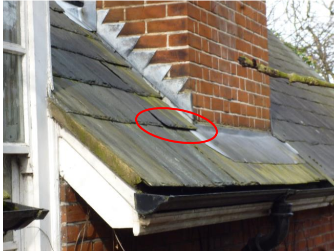
Photograph 7 TN1 - Lifted slate tile on the southern aspect of B1.
