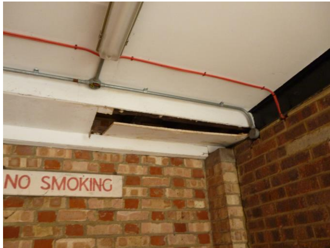
Photograph 8 TN2 - Broken soffit beneath the awning on B1.
