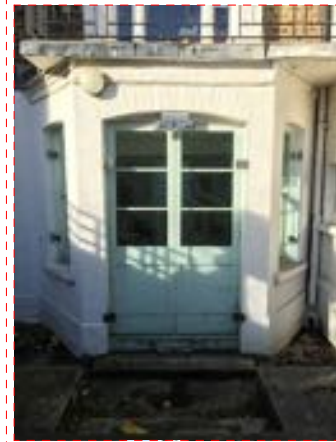
LGF extension door with the same style security glass as front elevation LGF windows.
