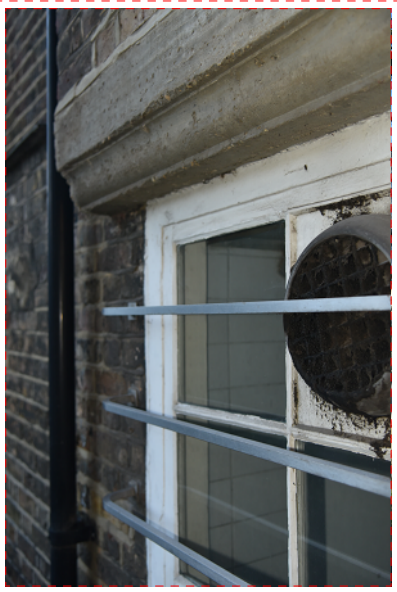
LGF kitchen window 1, kitchen fan installed through it.
