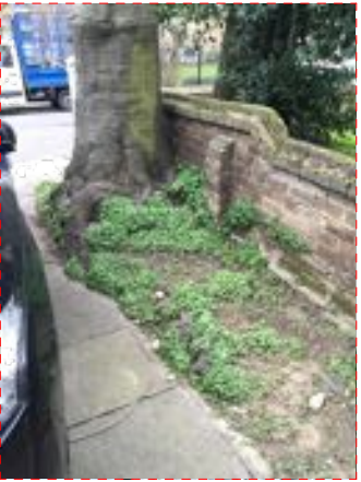
Facing north, the growth of old tree roots.
