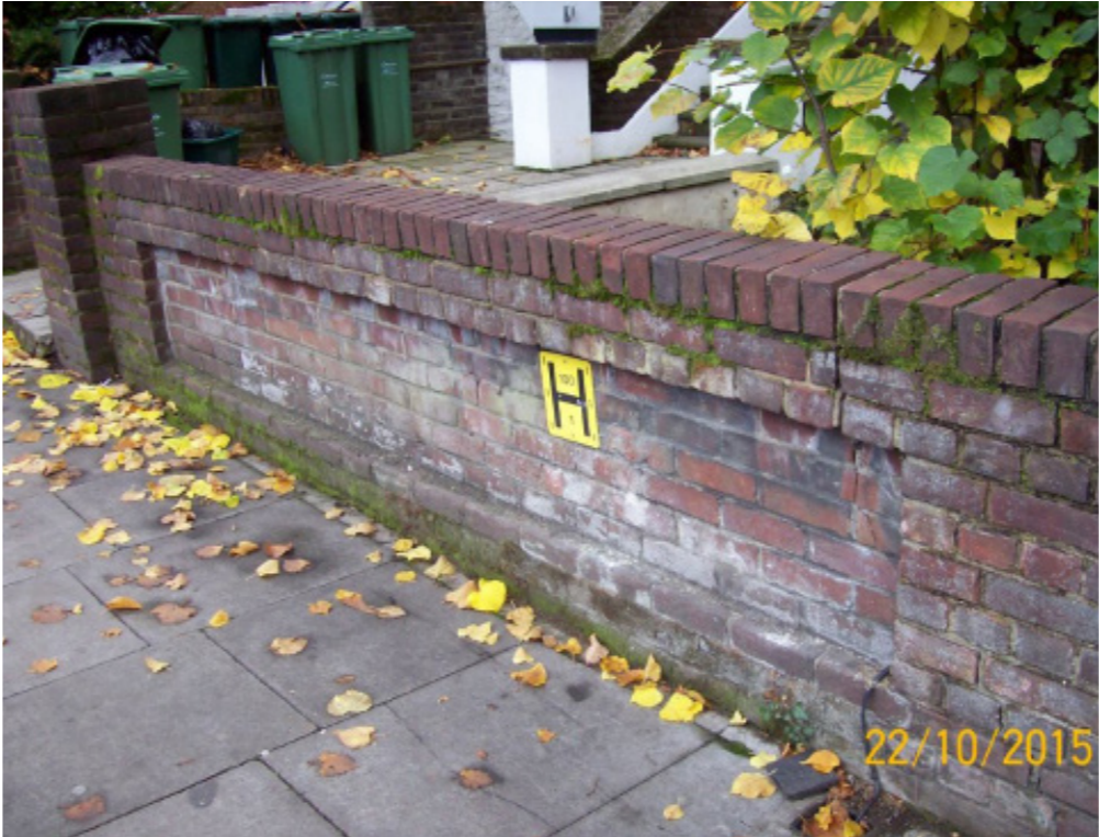
Street garden wall showing crack
