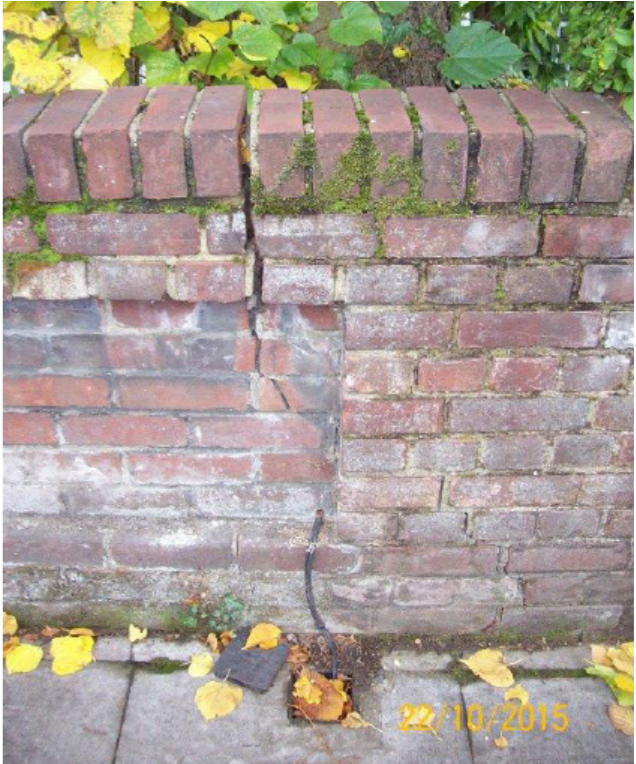
Crack in street garden wall
