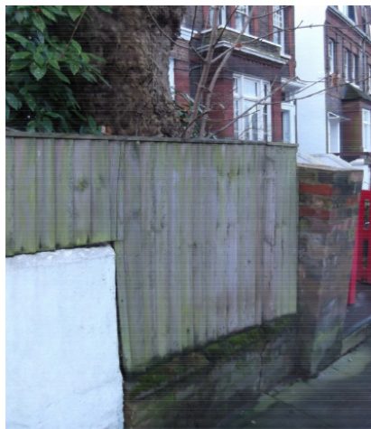
precedents in Broadhurst Gardens: front boundary walls replaced by fences etc due to proximity of tree causing issues with front garden walls
