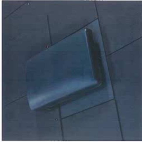
PHOTO 8 – Ventilation grill to bathrooms In roof, positioned behind chimney to mansard and London roof – not seen from either front or rear At ground level
