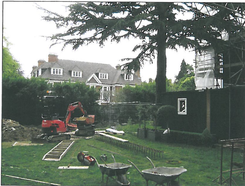
Photograph 1 – Mini excavator and mini dumper and pile of spoil on the lawn area. Protective boarding had been laid across the Root Protection Area. This must all be removed early next week and the protective fencing shall be put back and secured in position in accordance with the approved Tree Protection Plan.
