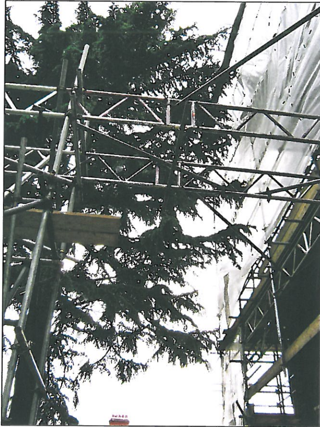
Photograph 3 – Looking up into the tree canopy and the scaffolding erected on the face of the building. There were no signs of any split or damaged branches. Scaffolding had been erected on the existing hard paved area.
