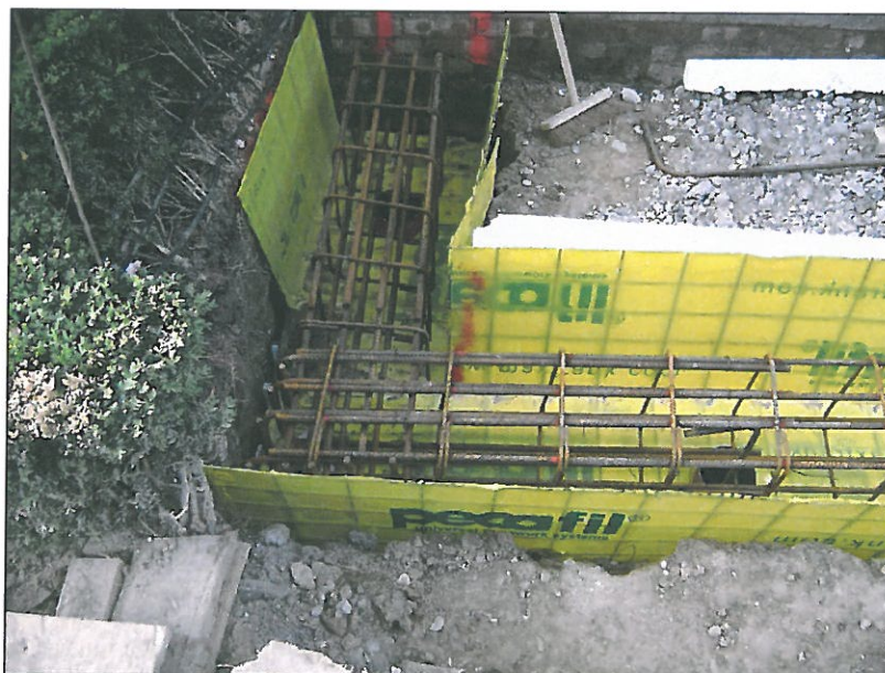
Photograph 2 – The excavation for the piles and reinforced ring beam foundation. There were no signs of any significant roots.
