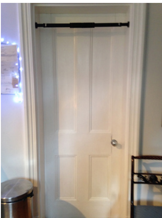
Figure 2: Existing historic door at lower ground floor level. The proposed new door to replace the basement flat entry door is to exactly match figure 2 in detail and materials.
