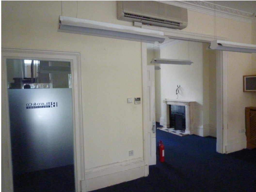
Fig.16 A view from the front to rear rooms on the first floor
