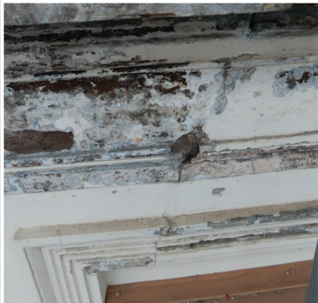
Fig 4. Old crack through mouldings
