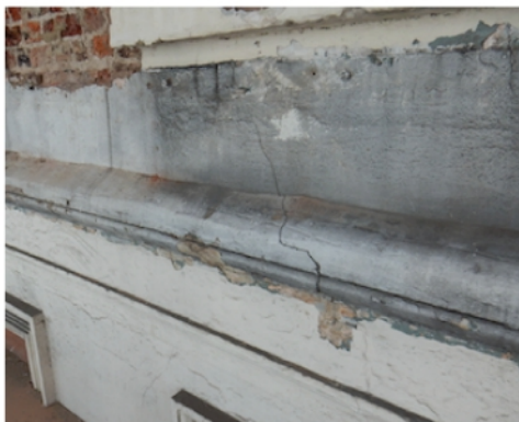
Fig. 3 Crack through rendered string course above window on the east elevation.
