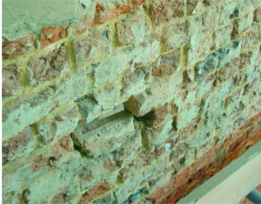
Example showing rough wall with loose bricks
