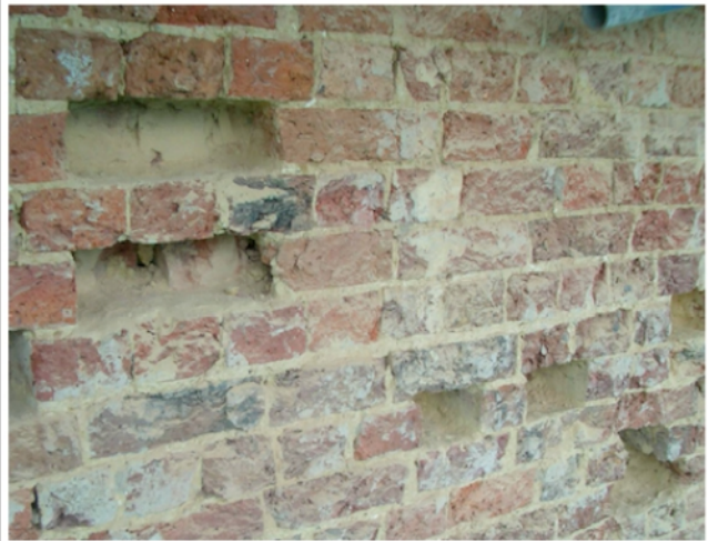
Example showing where defective or loose bricks have been cut out
