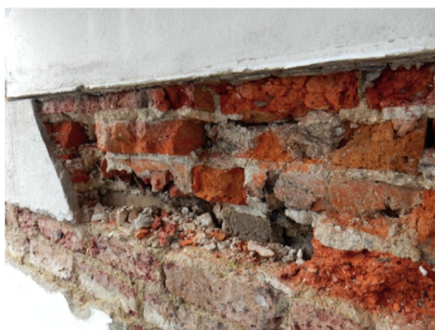
Fig. 6 Detail of poor brickwork
