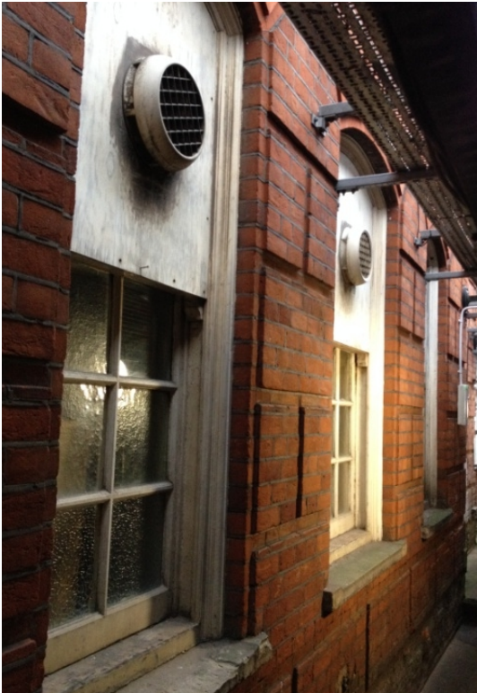
(image 5) Existing Windows view from the lightwell at basement level, at both of the affected windows.
