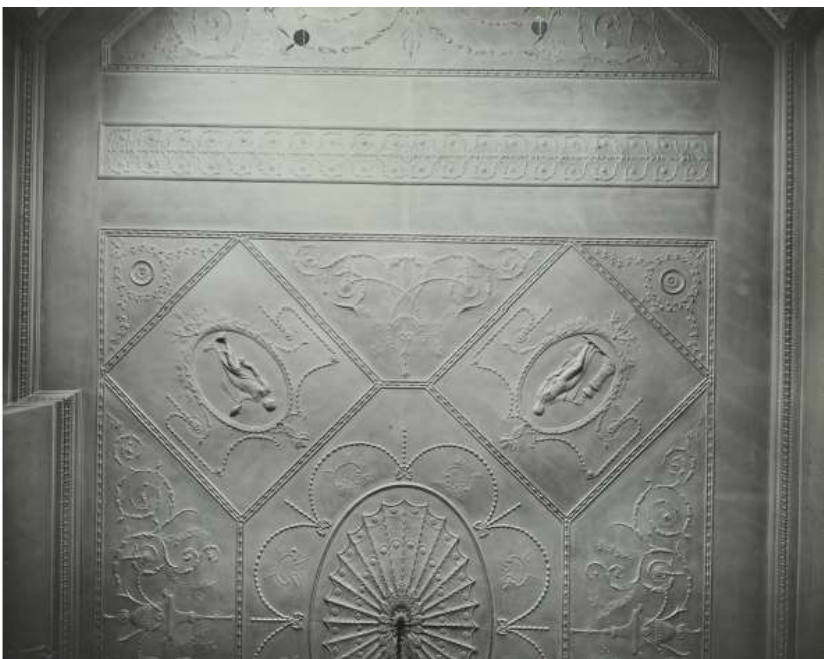
Picture 1 shows the ceiling of the rear room at first floor (from 1913)
