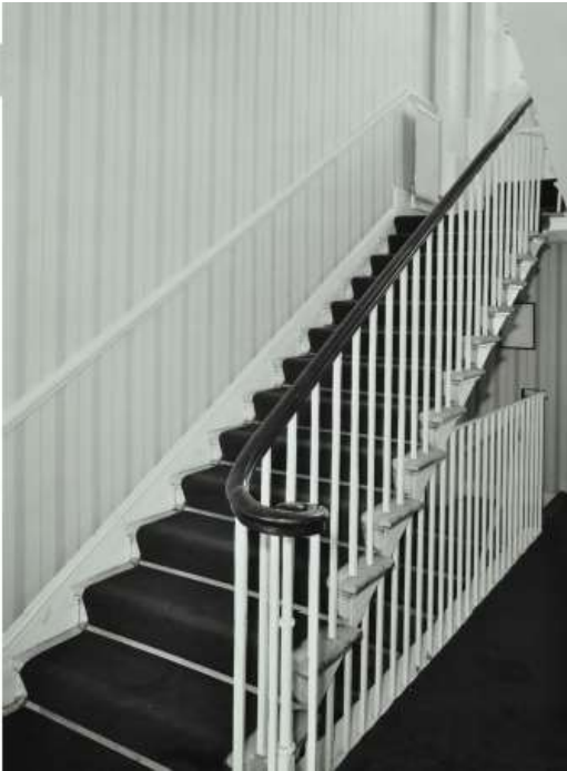
Picture 2 shows the plain cast iron balusters to the main stone staircase (from 1907)
